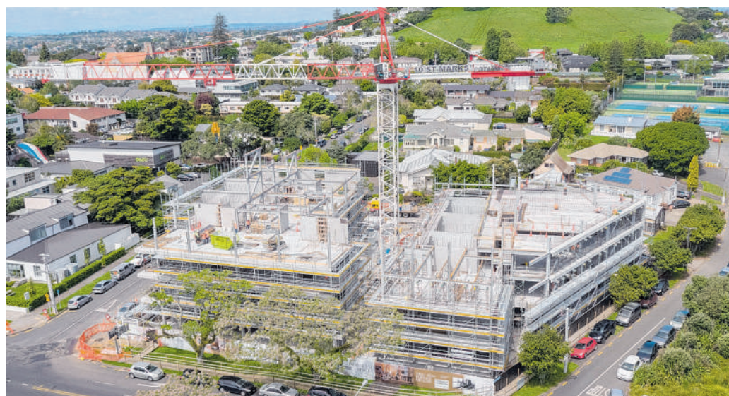
St Marks residential complex in Remuera received the first acknowledgement in the Innovation category of the Homestar Design rating system.
